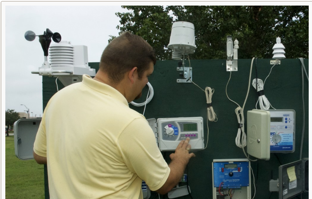
Charles Swanson, Texas AgriLife Extension Service landscape irrigation specialist, opens the programming unit of a ‘smart’ irrigation controller. Some of the different weather sensors manufacturers use on their controllers are mounted on top of the panel. (Texas AgriLife Extension Service photo by Robert Burns)
