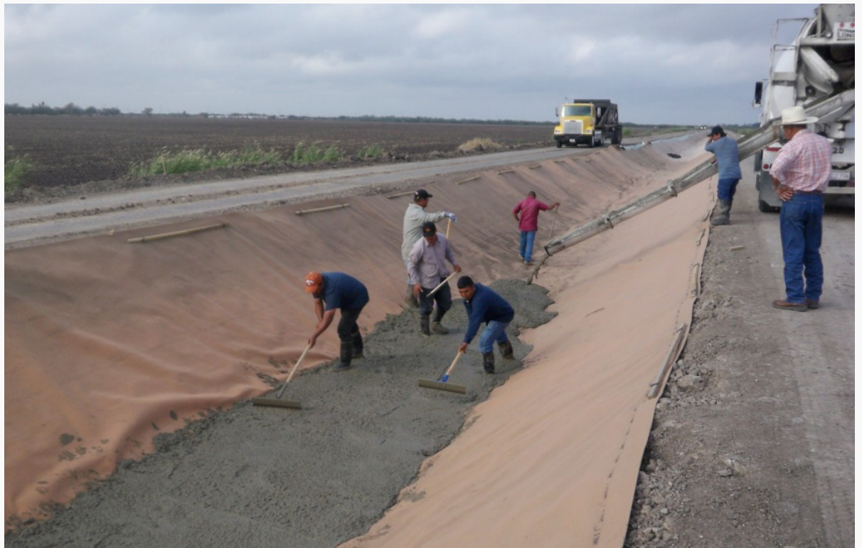
Workers in Hidalgo County spread concrete over a synthetic canal liner made of polyester. (Texas AgriLife Extension Service photo by Askar Karimov)
